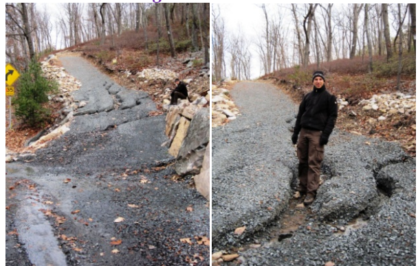
Damage to the launch road
